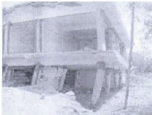
Fig. 1.4 Beam-Column joint failures
