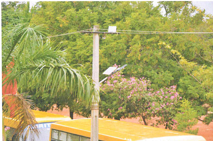
Solar Panel for the electrical poll light
