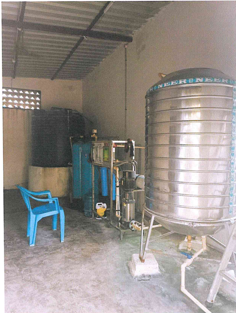
RO Plant Water Plant
